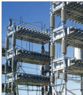
Open Rack Harmonic Filter Bank
