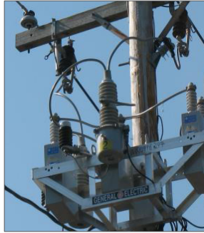
Pole Top Shunt Banks
