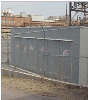
Metal Enclosed Shunt or Filter Bank
