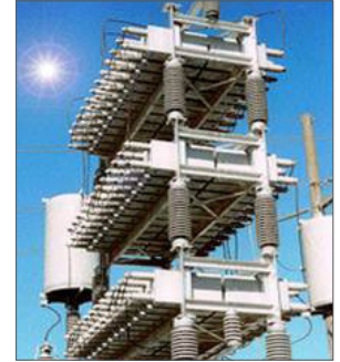
Open Rack Shunt Banks
